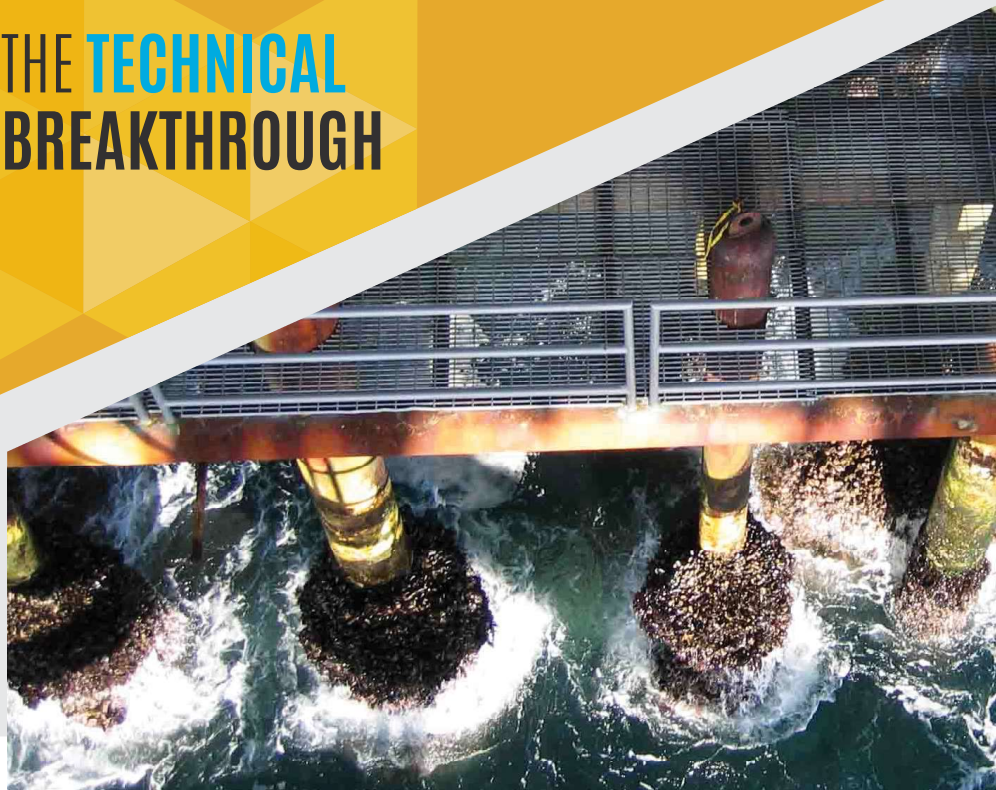
Prolific marine growth on offshore structure
