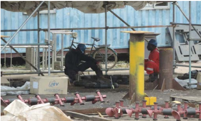
Prior to installation, the MGP products assembled and tagged with the assigned jacket members at the yard.
