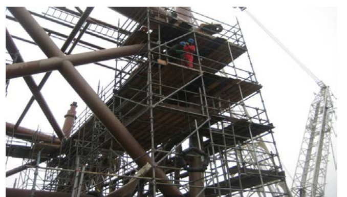
Despite the obstructions on the jacket structure, using rope, the MGP products were lifted up and installed at the designated members.
