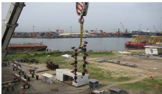
At some areas of the jacket, the MGP products were also installed using crane and cherry picker.
