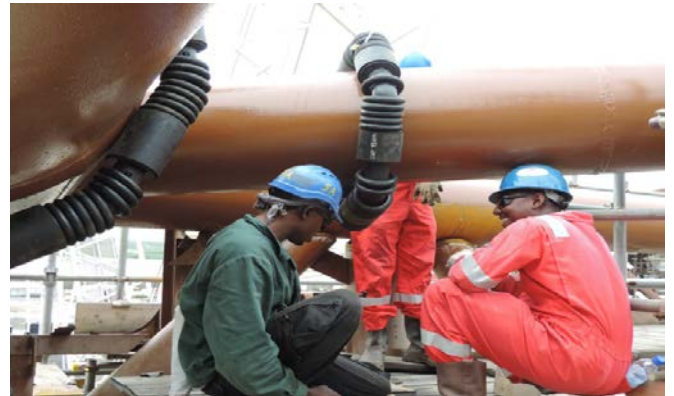
The tagged MGP products were then, installed onto the assigned jacket members.
