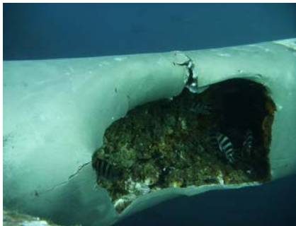
5. Defect on structural member
