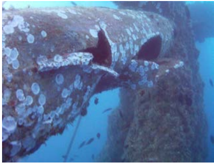
1. Defect on structural member
