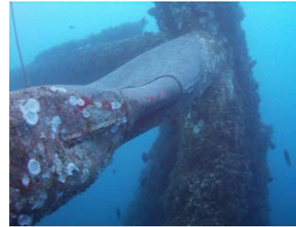
3. Defect on structural member
