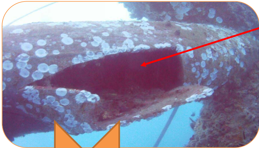
Tear in member at 11 m of water depth
