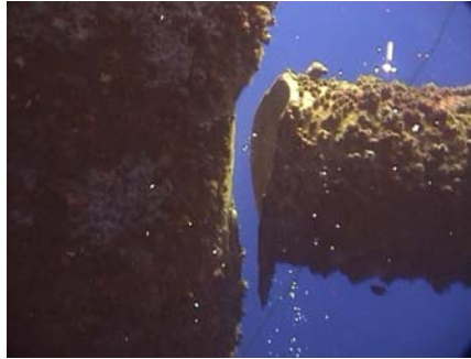
1. Damage at main leg
